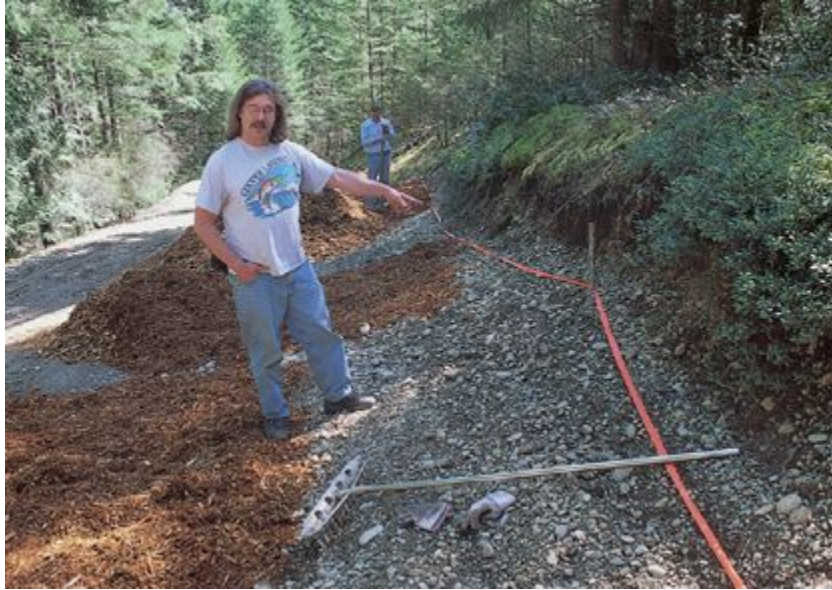
FIGURE 92 David Sumerlin points to location where wood chips should be placed—up against the bank of the scar face of the road cut, thus eliminating erosion from the silt-producing exposed surface.
